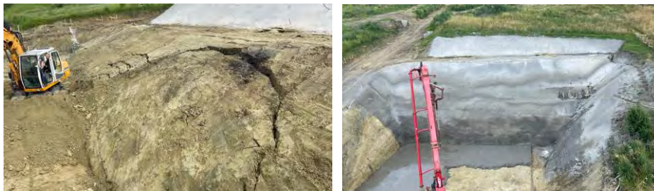
Figure 4: Final excavation unconsolidated and locally failed (left) and consolidated by soil nailing technique (right)
