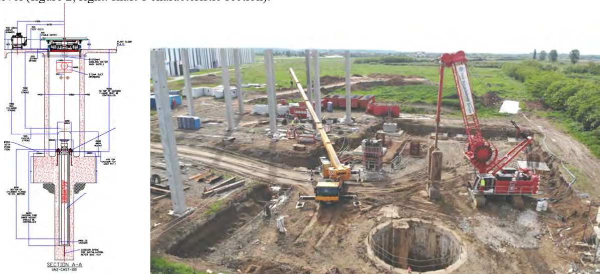
Figure 1: left: technical concept – vertical casting machine (VCM), right: photo during circular shaft construction
